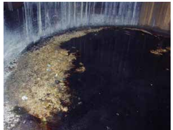
Stack Corrosion Inspection
