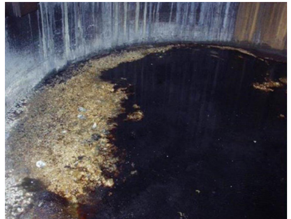
Stack Corrosion Inspection
