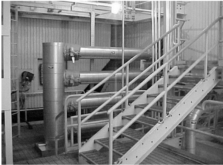
Figure 2 Dilution air and ammonia injection to SCR reactor
