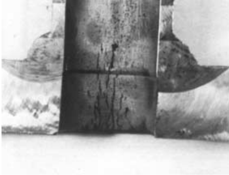
Figure 2 Sample Piece of Economizer Inlet Header Showing Cracking in Header Bore Hole and Tube Connector
