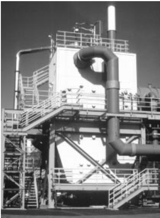
Figure 3 The 100 million Btu/hr (29MW t ) U-Fired Test Facility
