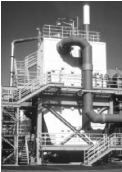
Figure 5 The 100 million Btu/hr (30 MW t ) U-fired Test Facility
