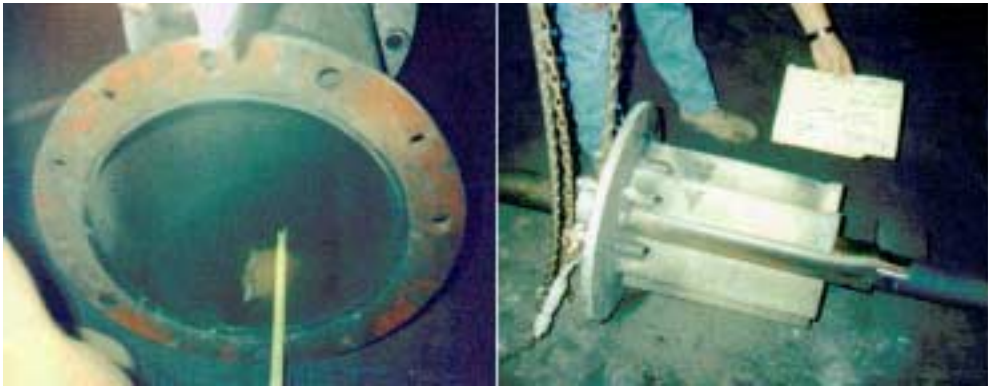
Figure 4 Field documentation of erosion in coal burner spool piece and head vanes.
