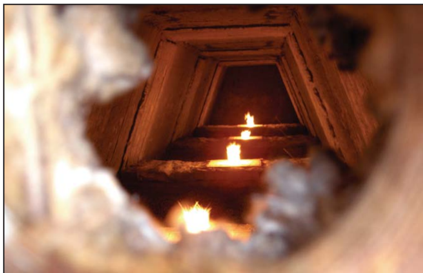
Figure 7. Photo of burners taken from view port of a 5 Canister RSCR system.
