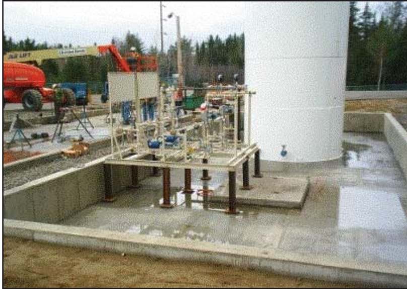
Figure 8. Ammonia skid with storage tank for a 50 MW boiler.
