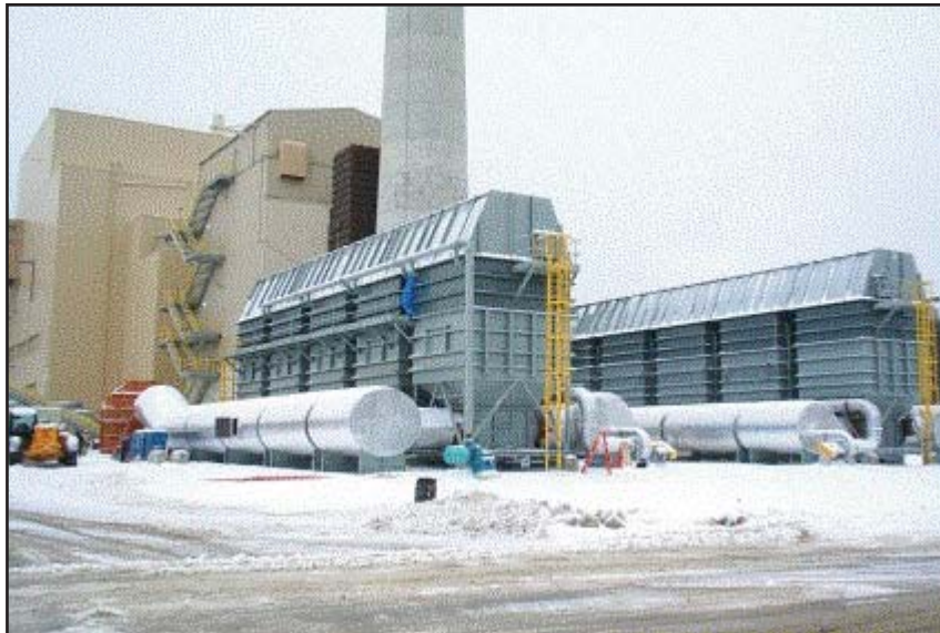
Figure 11. An RSCR system showing two trains of 5 canisters each.
