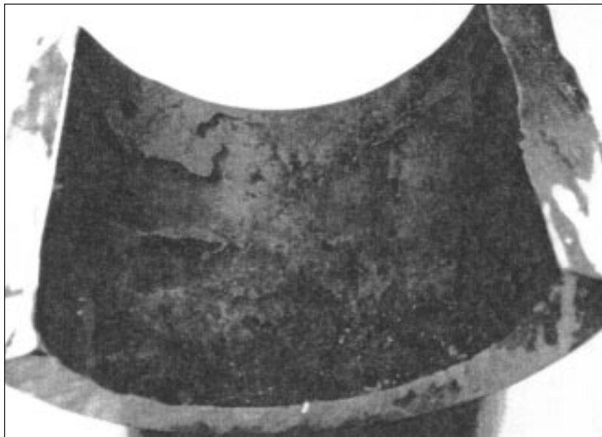
Figure 6 Typical example of a piping section with evidence of flow accelerated corrosion on the inside surface.
