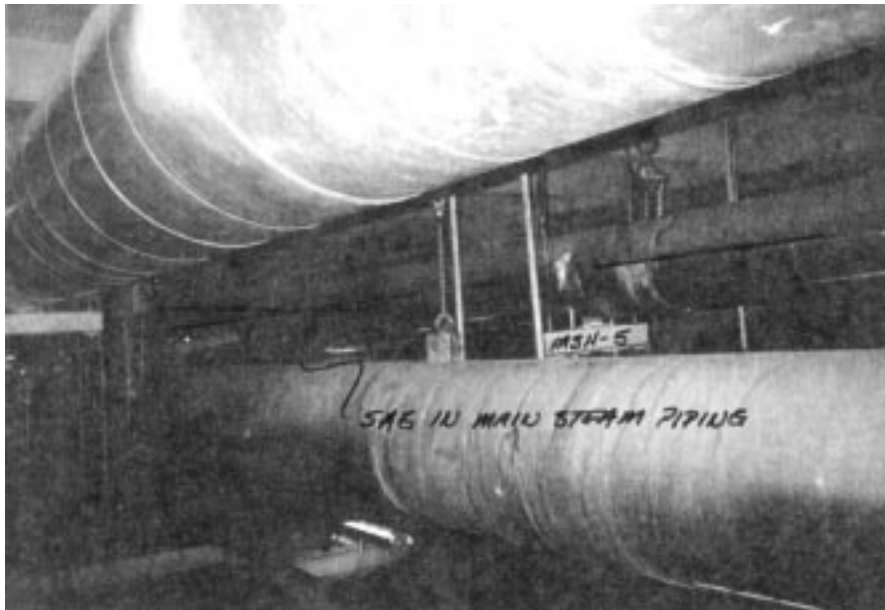
Figure 1 Main steam piping general view of sagged horizontal portion.
