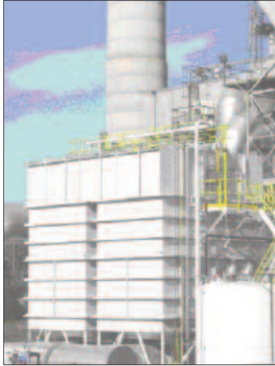
Figure 7. An installed two canister RSCR System on a 15 MW unit
