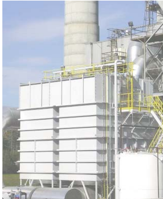
An installed two canister RSCR System on a 15 MW unit
