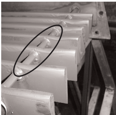
Figure 6 - No protective cladding on the flow element
