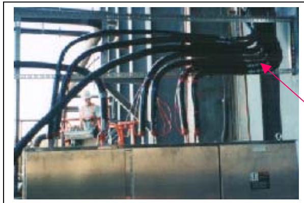
INSIDE RADIUS TOO TIGHT
