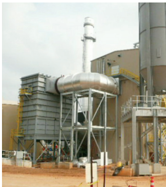
▲ ETEC's Hilton Lively Renewable Power Biomass Project in Woodville, TX
