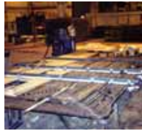
Replacement Reheaters for Existing Unit
